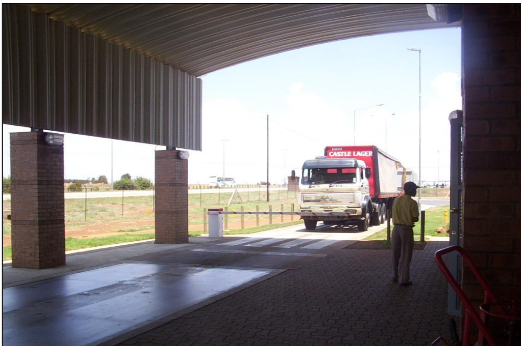
N4 weighbridge facility in Middleburg, where Weighbridge module of the TRAFMAN™ system is installed and operational.
